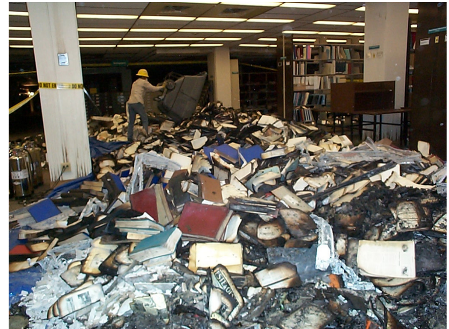
Fire damage at the University of New Mexico Library
